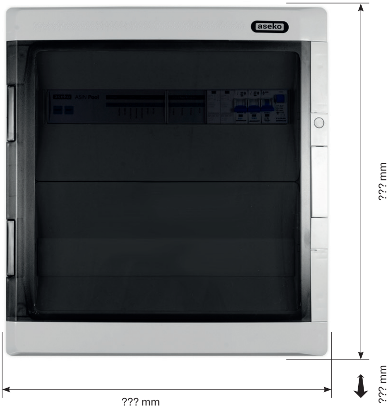
ASIN Pool Electrical Box # 12168
